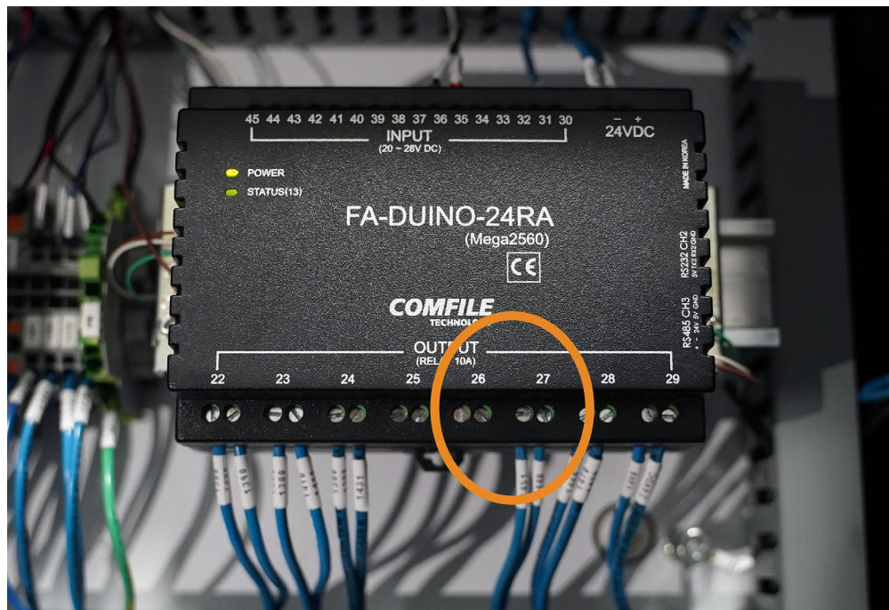
VariFlow PLC alarm signal
